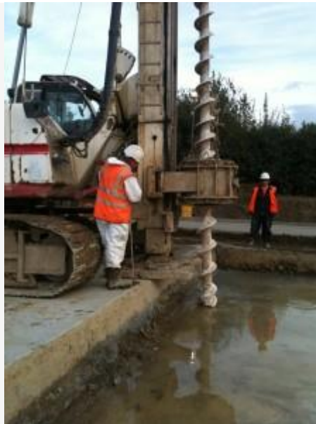
Auger piling on two tier RoadCem mat, note no shear problems at all
