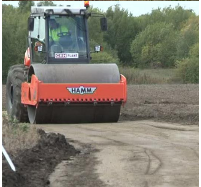
Picture 1: National Grid temporary Road Trials at Brinkworth, Nr Rotherham by AMEC
